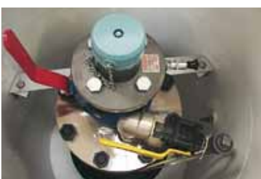
Typical Low Point Drain Equipment Installed
