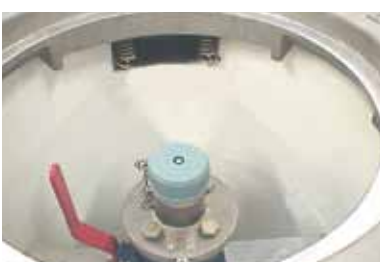
Typical High Point Vent Equipment Installed
